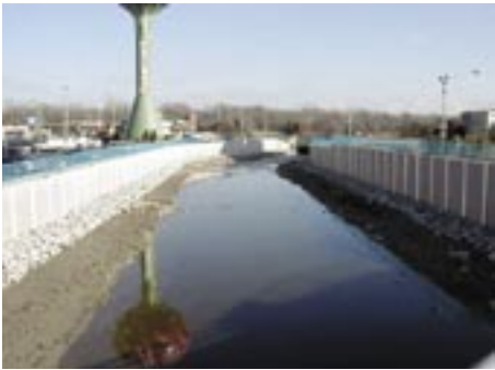
Floodwalls along Willow Creek in Rosemont, Illinois. Source: Kevin D. Richards, U.S. Geological Survey.
