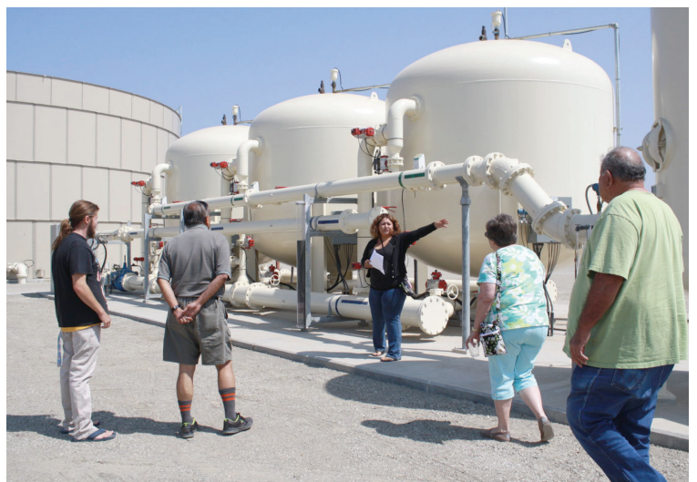
The Armona Community Services District received funds from Prop. 1 and the State Water Resources Control Board to fix long-standing water quality issues.
