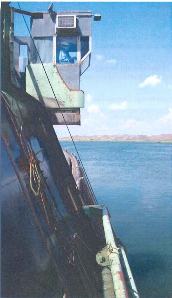
Vito Palumbo, IID water construction worker, operates the trashrack at Imperial Dam.
