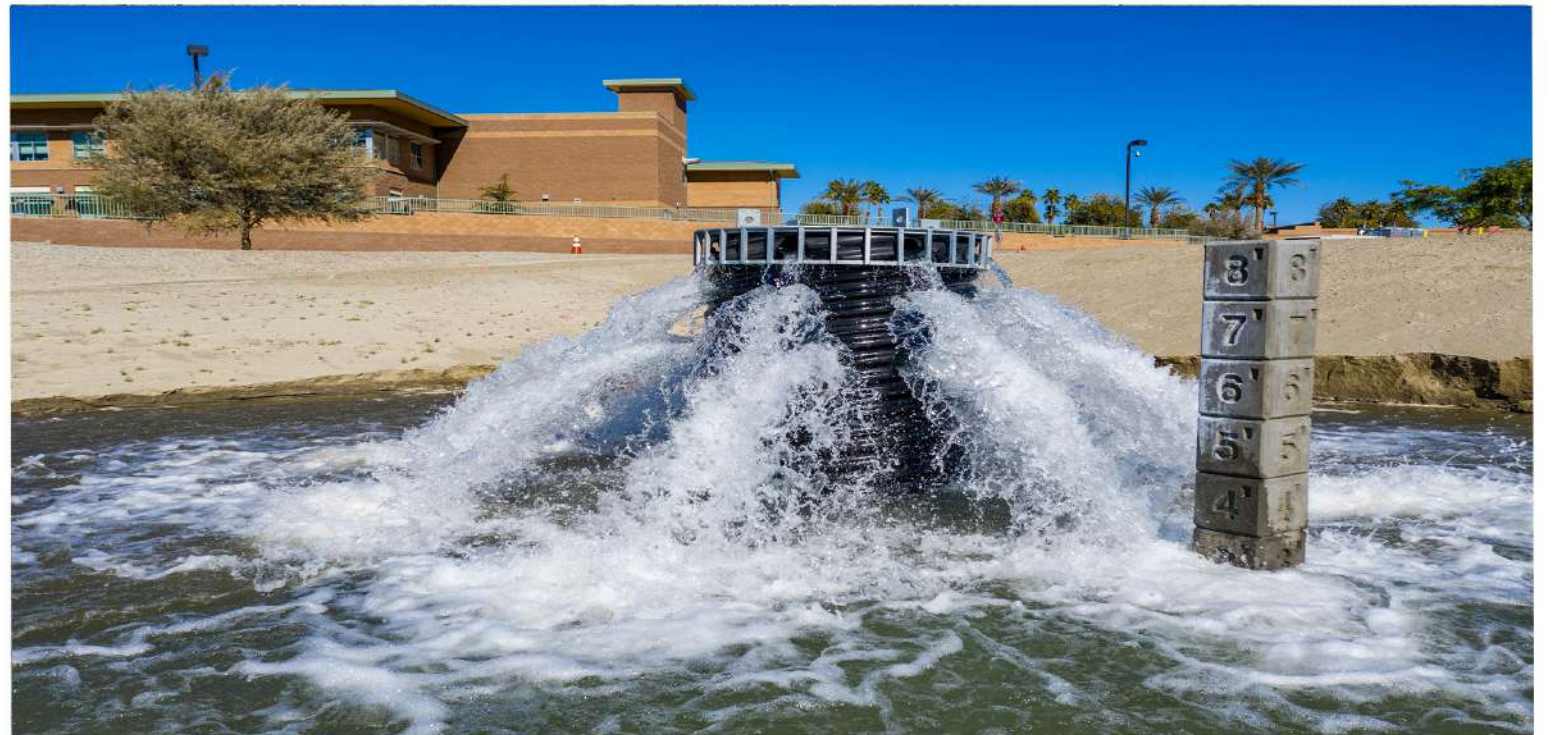
On February 20, 2019 CVWD celebrated the completion of Phase 1 of the Palm Desert Groundwater Replenishment Facility. When fully completed it will percolate an additional 25,000 acre feet of imported Colorado River water into the Mid-Valley aquifer each year.
